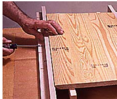
3--Use drywall screws to secure the work to the tracks. Stepped blocks shown in the drawing (left) hold work at correct height.
